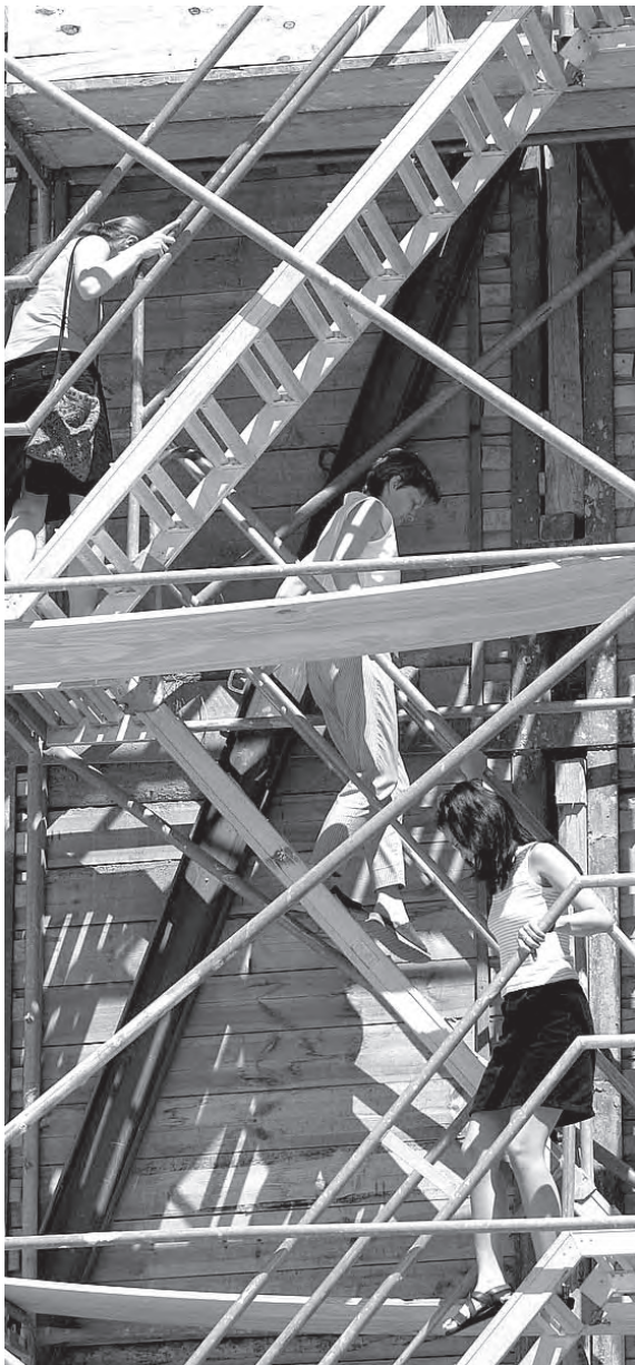
Others dare to descent into the excavation pit. Andere wagen den Abstieg in die Baugrube.
