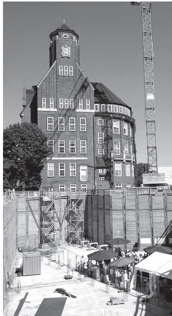
A hot summer day on the construction site. In 2007 this site will harbour a modern research infrastructure with specific-pathogen free animal husbandry, an insectary and biological safety laboratories up to level 4.
